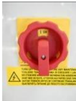
Picture 17 – Main switch ON
