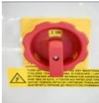
Figura 17 – Interruptor general en ON
