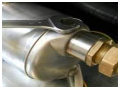
Figure 15 – Purge de la pompe
