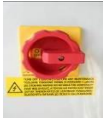
Picture 7 – Main switch
