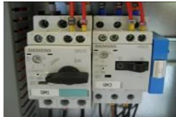
Picture 8 – Circuit breakers
