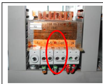
Picture 5 Transformer set at 400V
