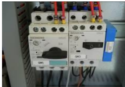
Picture 16 – Pump breaker ON
