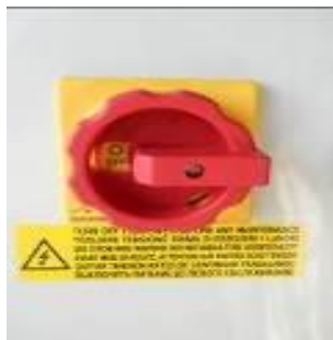
Figura 7 – Interruptor general OFF
