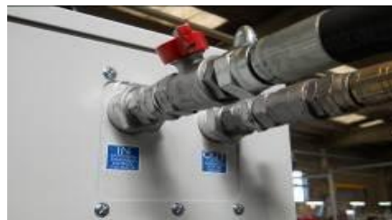
Picture 13 – Pipe connection
