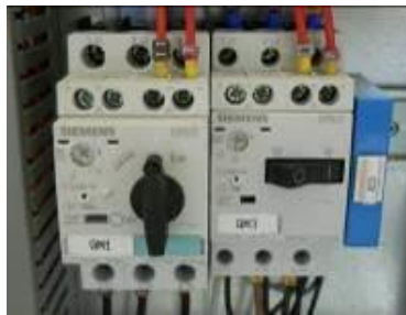
Picture 20 – All circuit breakers ON
