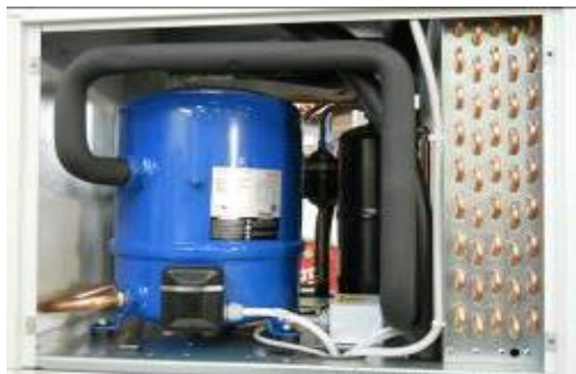
Picture 22 – Compressor placement
