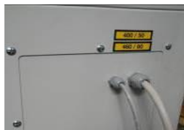
Picture 14 – Electrical connections
