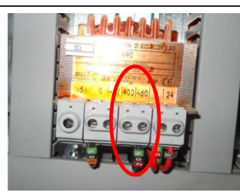
Picture 6 Transformer set at 460V
