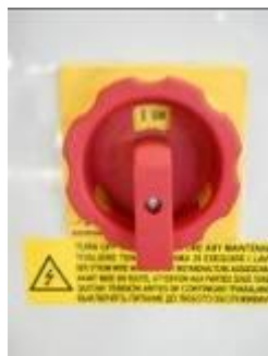
Picture 16 – Main switch ON
