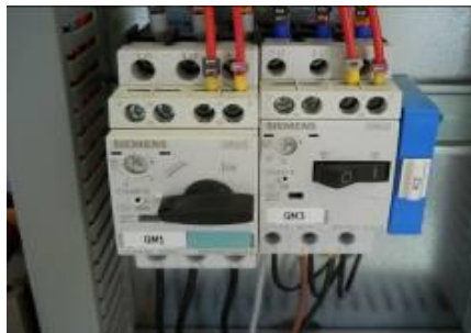
Picture 15 – pump breaker On
