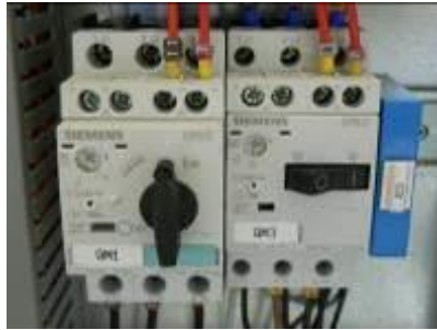
Picture 19 – All circuit brakers ON
