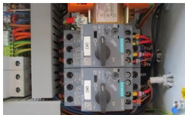
Picture 12– pump breaker On
