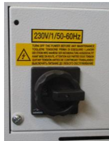
Picture 7 - Main switch
