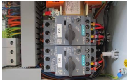
Picture 8 - Circuit Breakers
