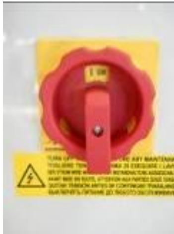
Figura 13 – Interruptor principal ON
