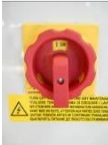
Picture 13 – Main switch ON
